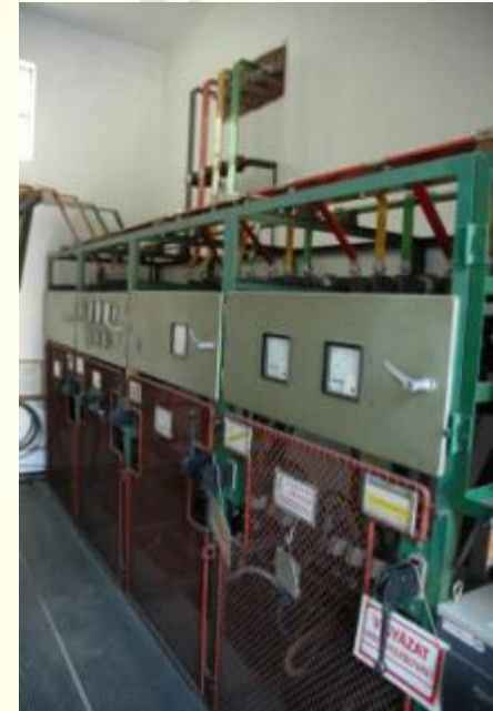
0.4 kV distribution box
