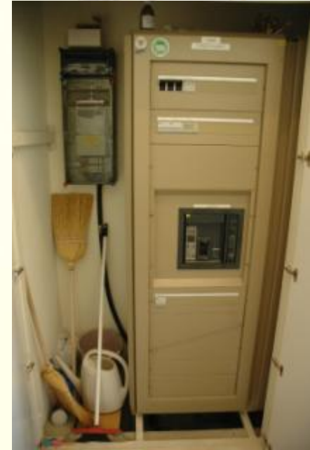
0.4 kV main supply
