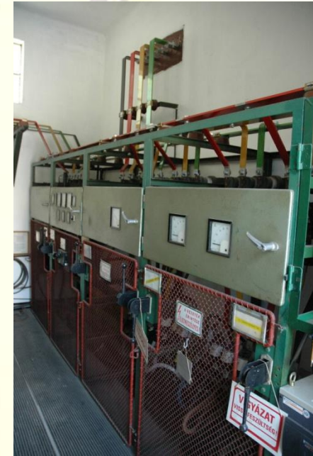
0.4 kV distribution box
