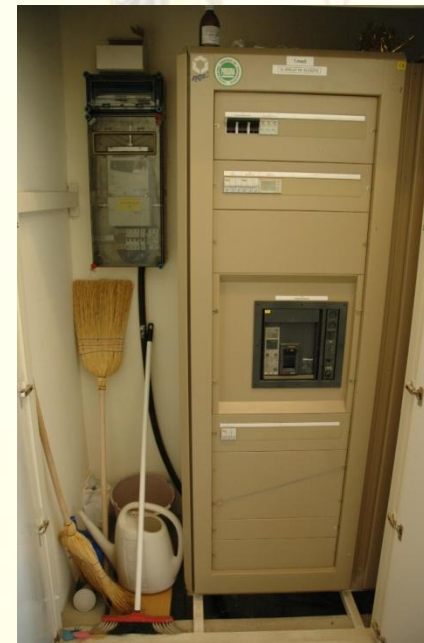
0.4 kV main supply
