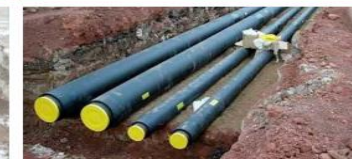
New heating and cooling system
